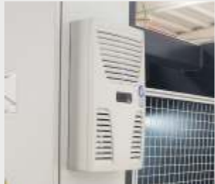
Electrical Cabinet Cooling System
